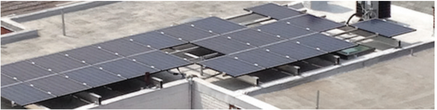
Metal beams that span the width of the home are a common way to mount solar on row homes with flat roofs
