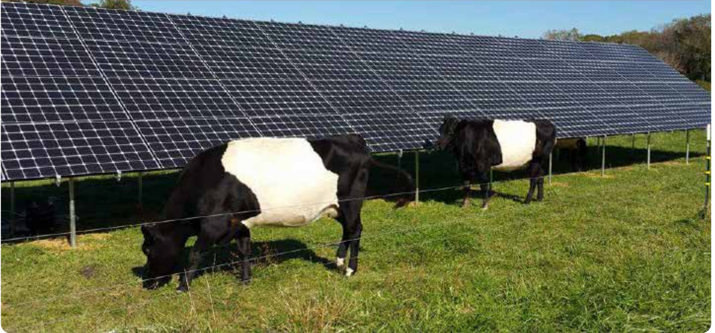
Cows graze aside a ground mount solar installation.
