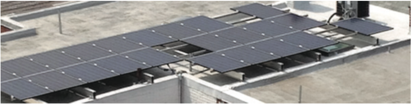
Metal beams that span the width of the home are a common way to mount solar on row homes with flat roofs
