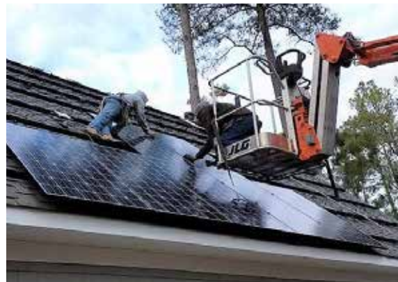
Solar Installation. (Courtesy of Shockoe Solar).
