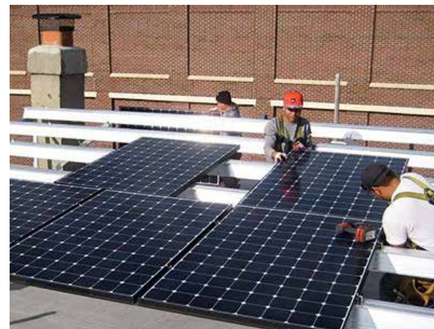
Solar installation, courtesy of Thomas Burnett.
