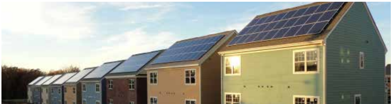
Installations on a group of new homes in Virginia. Image courtesy of Alt Energy.
