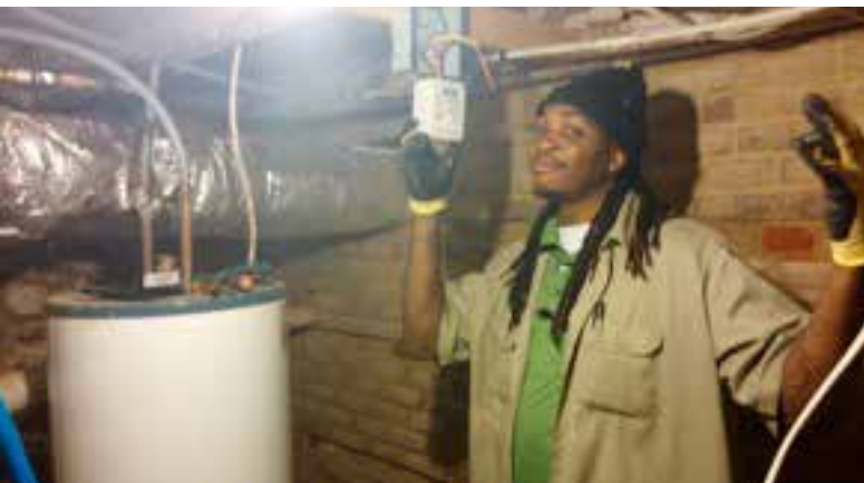
Local electricians installed regulators on hot water tank in Shepherdstown as part of the Shepherdstown Solar Holler project
