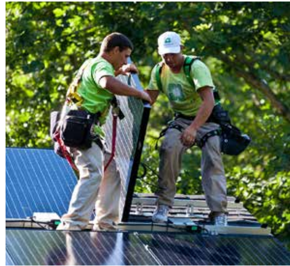
Installers put up systems as part of the University of Maryland solar co-op
