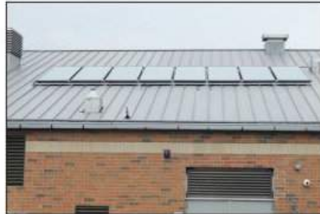
Northwest Local Elementary School solar thermal collectors
