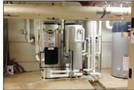
Northwest Local Elementary School's solar heat exchanger and hot water tanks for preheating water to add to the boiler, as needed.
