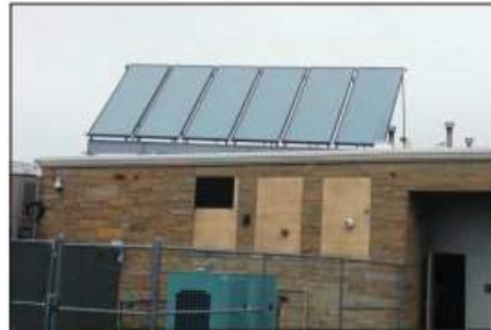
Northwest Local Middle School solar thermal collectors
