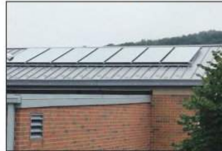
Northwest Local High School solar thermal collectors
