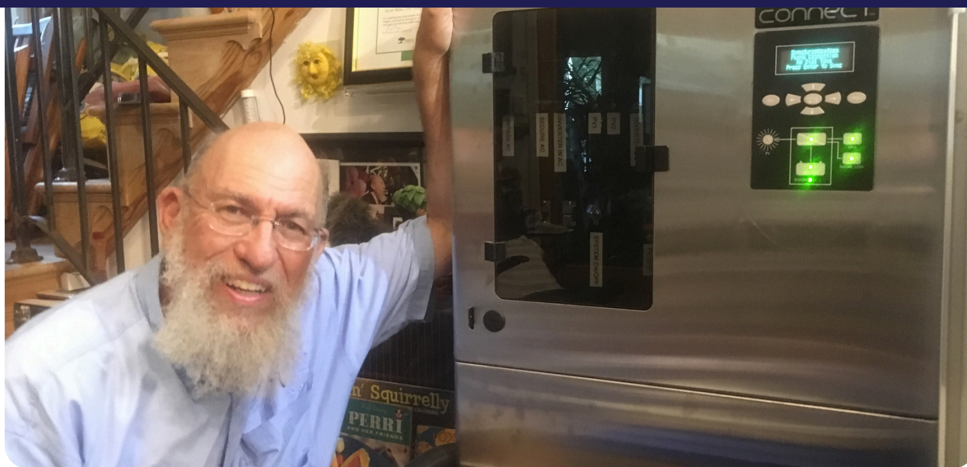
Virginia homeowner Scott Sklar with his GridPoint Connect battery.
