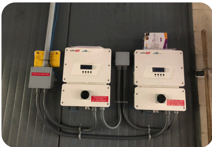
Two grid-tied inverters on a solar home in Florida.
