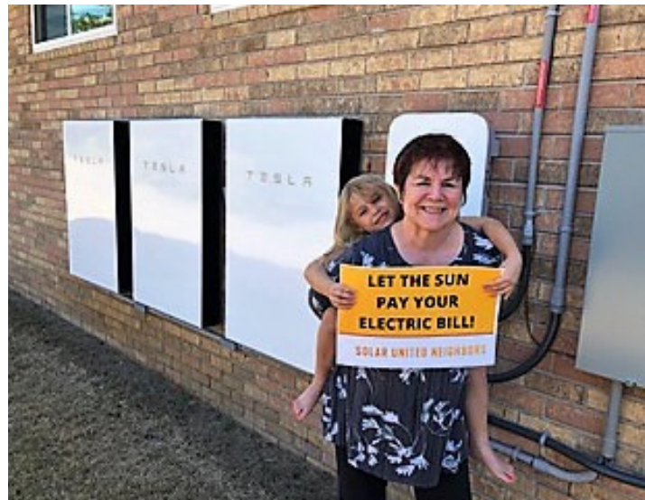
Florida homeowner Mary Blackwell and child with her Tesla Powerwalls installed.
