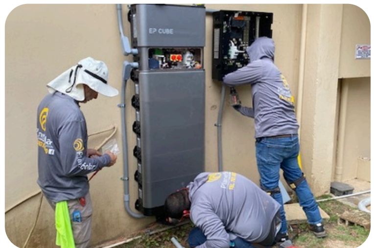
Installation of 8.1kW system in Centro Buen Pastor, in Barrio Rio, in Guaynabo—February of 2024.
